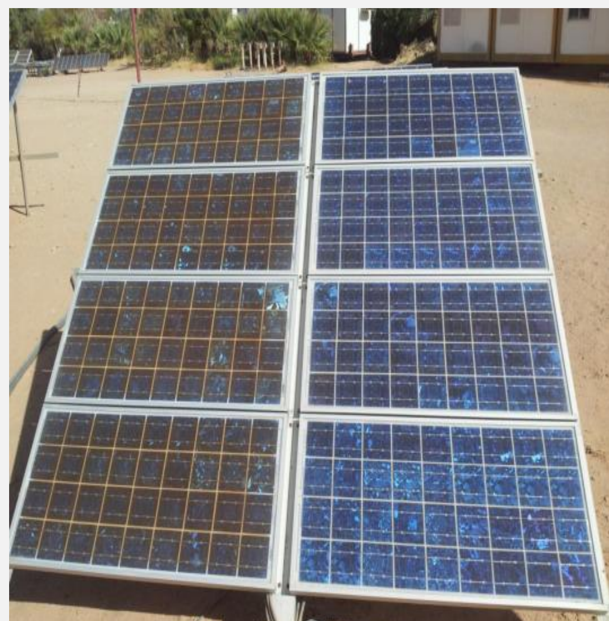
Outdoor multi-c-Si Module showing yellowing and metalization corrosion. (N.kahoul et al, reneue 2017)
